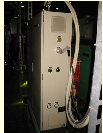
Energy extraction switch, Tested in TCC2
