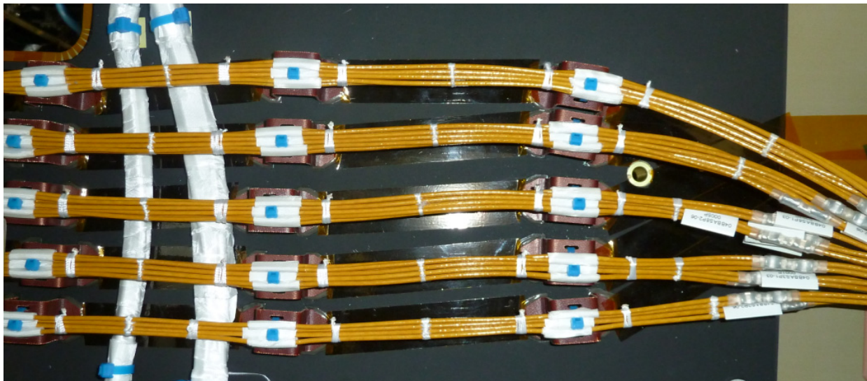
Fig. 5: High power Satcom harness split in five AWG12 flat bundles to reduce the derating factor.
