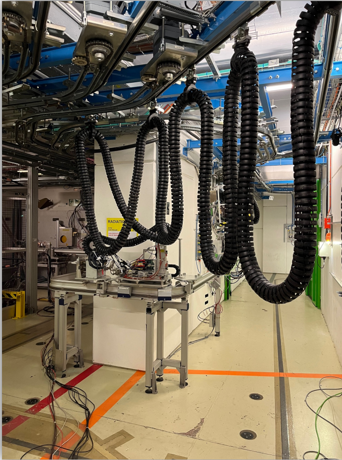
The Montrac conveyor connected to the patch panel with a cable chain.
